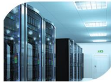
DATA CENTRE FUEL TESTING
